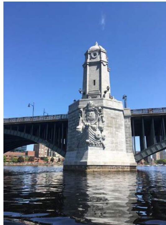
Rehabilitation of the historic Longfellow Bridge was completed in 2018, and reopened to traffic between Boston and Cambridge.
