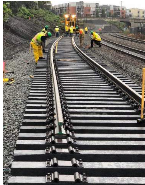
Crews relocated commuter rail tracks in Somerville to create space for the Green Line Extension tracks.
